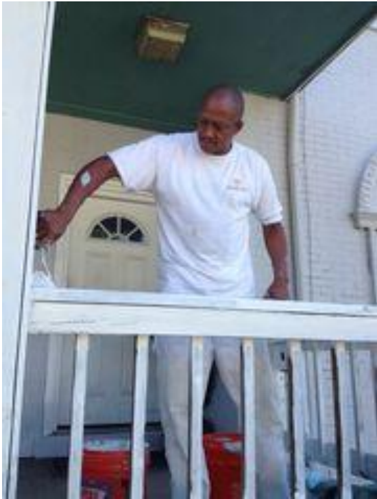
Cal Barrett, 50, a contract painter, puts primer on the porch at 3568 Bogart Ave., Avondale, as part of an overall street cleanup and restoration. (Photo: The Enquirer/Mark Curnutte )
